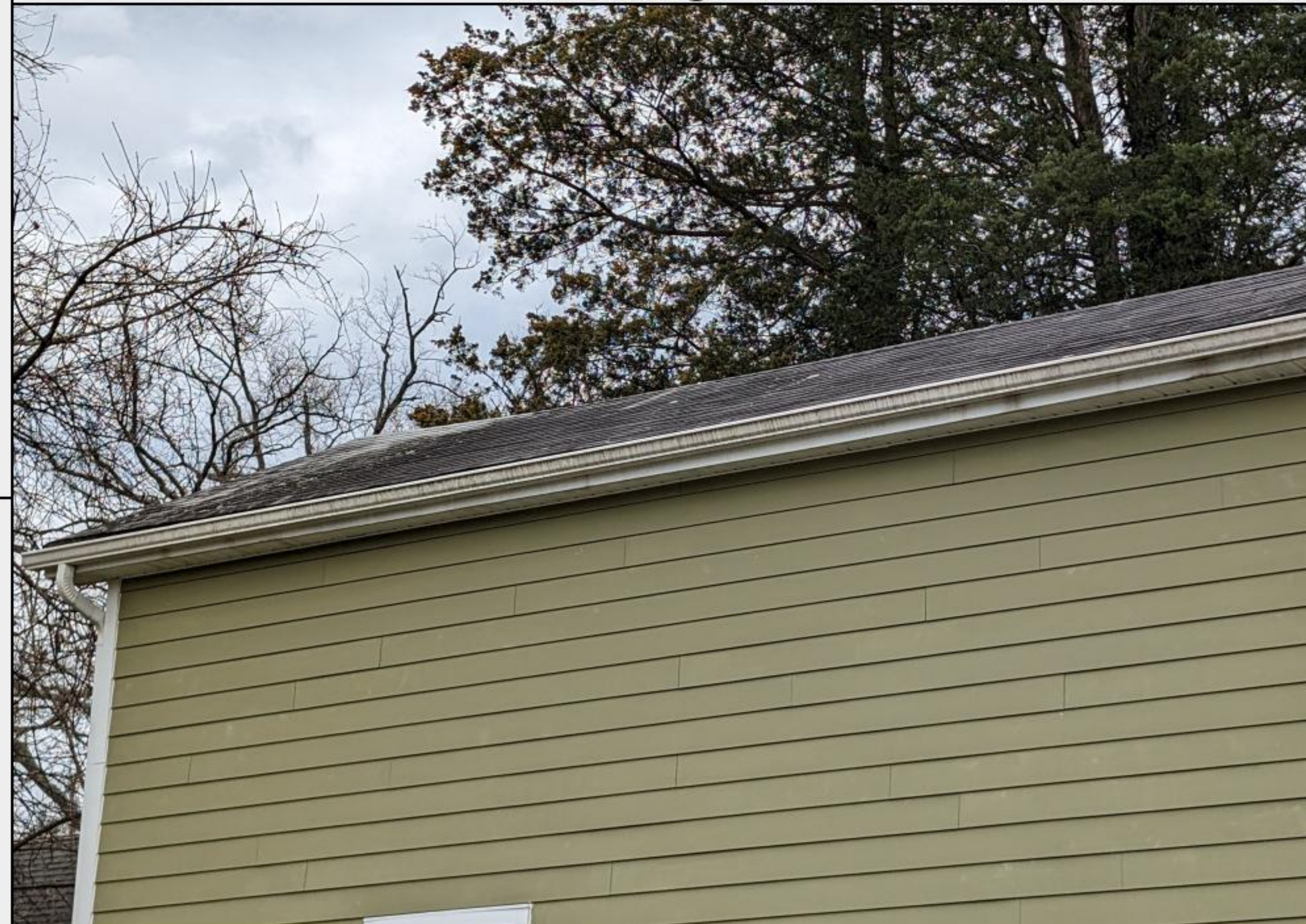
It needs a new roof
