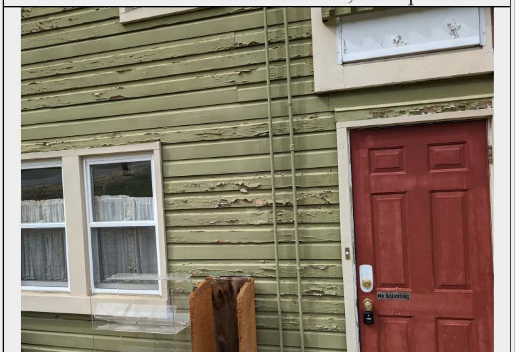
Paint in bad shape
