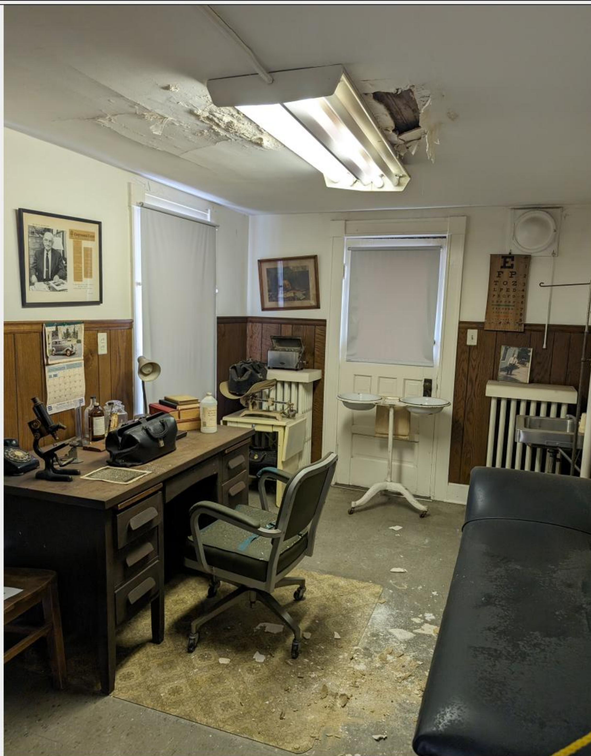
Dr. Brumbaugh's Office - notice crumbling plaster
